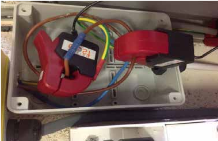
Example of a junction box protecting the current sensors
